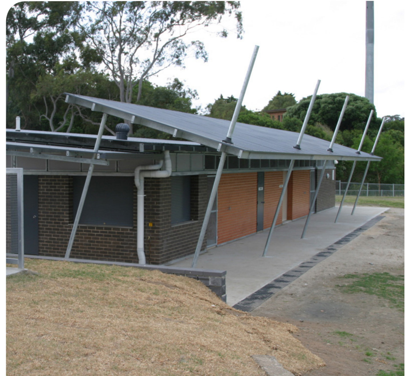
A new amenities block was constructed at Picken Oval, Croydon Park this year.
